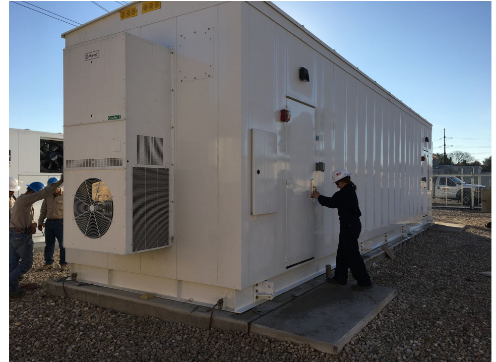
Battery at Austin Energy's Kingsbery Substation
