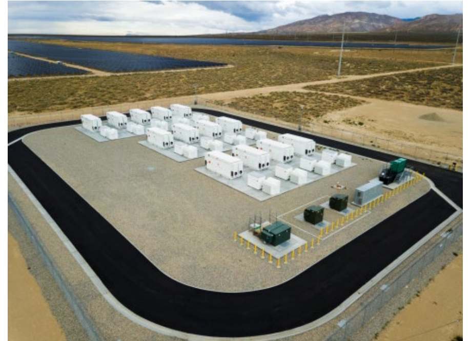
LADWP's 20 MW energy storage project in the Mojave Desert
